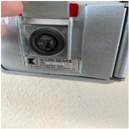
Knox box located next to lobby door
